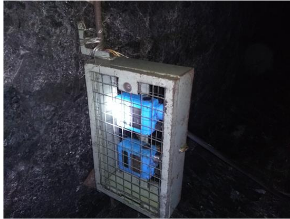
Fig 7: Gas sensors installed in the BG panel for continuous monitoring of goaf atmosphere at GDK 11 mine
