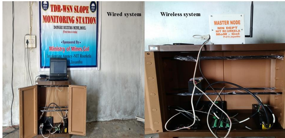
Fig.7. Installed TDR instrument in Protecting Room at mine site
