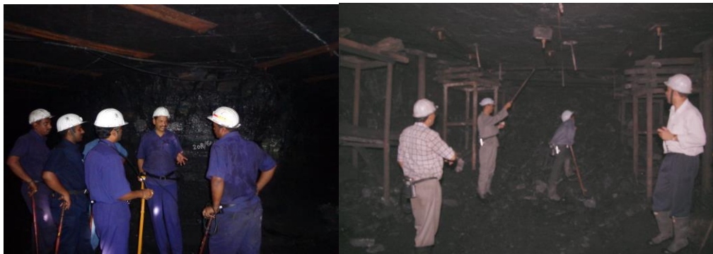
Fig 1: Status of pillars in typical underground coalmines prone for cracks and failure
