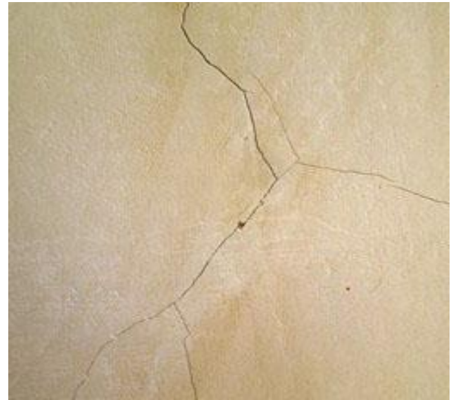
Fig.3 Original Wall image showing a hairline crack
