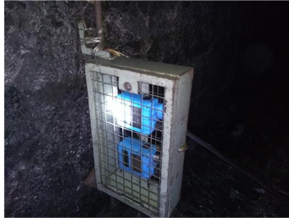
Fig 7: Gas sensors installed in the BG panel for continuous monitoring of goaf atmosphere at GDK 11 mine
